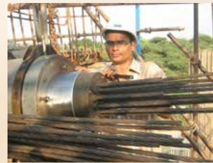
Measurement of Elongation in HT strands in Pre-stressed Box Girder of Flyover
