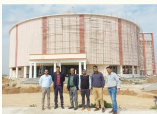
Construction of VC & Administration Building for Lala Lajpat Rai University for Veterinary and Animal Science at Hisar, Haryana
