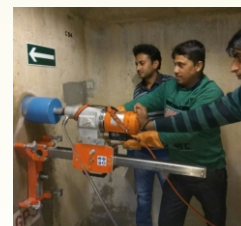
Extraction of Concrete Core of 150 mm diameter from Gallery Portion of Dam structure
