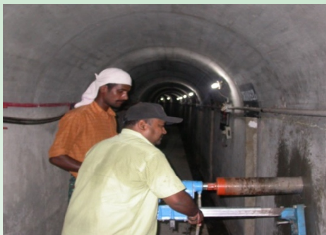
Concrete Core extraction of 150 mm diameter & 1 metre length from gallery of Gravity Dam
