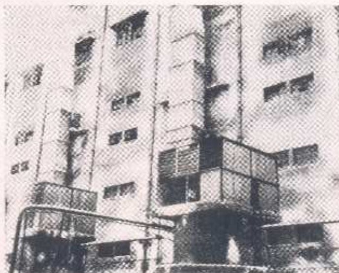
Fig. 1 Exterior walls with discoloured patches
